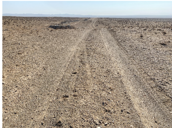
Figure 10: Access Road condition in a few areas
