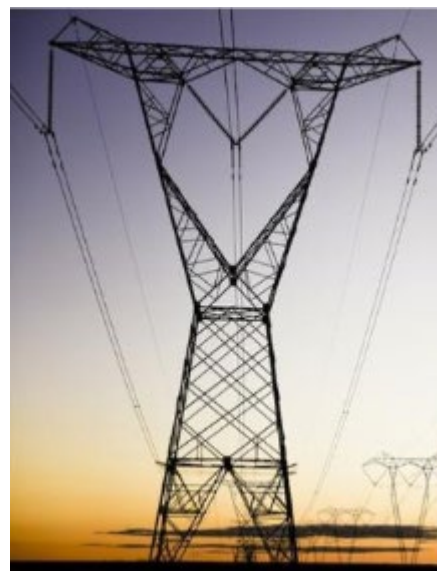
Figure 8: Self-supporting 500 kV Steel Lattice Suspension Tower (single circuit) (source: NEGU)
